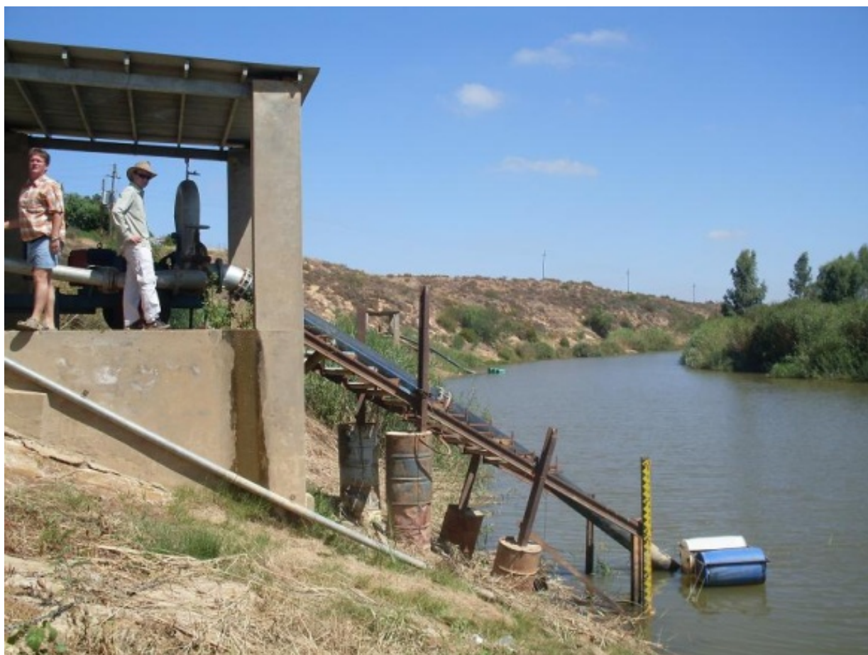
Addendum Figure 2 Morester Pump station
